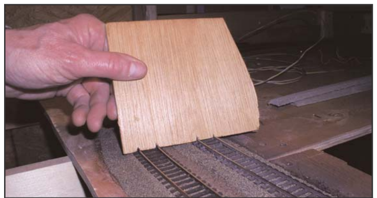
A spacing gauge is used to make sure tracks are laid parallel to one another.
