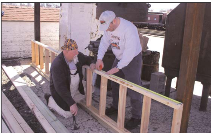
Mike Miciukiewicz and Skip Kern, who are blacksmiths and volunteers at the DRM, worked for many days to erect a frame, then cover it with sheathing for the forge. Mike installed the electrical system including lighting. Glenn Miller assisted them. Carolyn Taylor stained the sheathing. Mike and Skip were instrumental in recruiting other blacksmiths to participate in the Hammer-In, and in publicizing the event.
