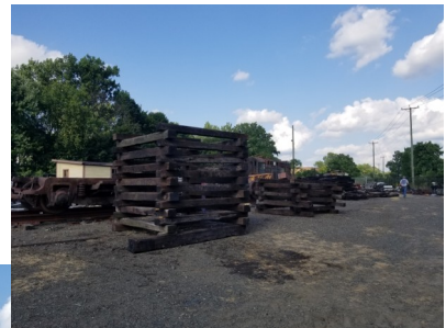
Above: Here, we see the completed cribbing. The top of the arch will lay on the smaller stack, with the braced end laying on the taller stack to prevent damaging the diagonal angle iron supports.
