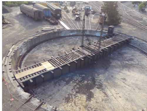
Left above: Aerial photo of the redecked turntable. Photo by Justin Chapin.
