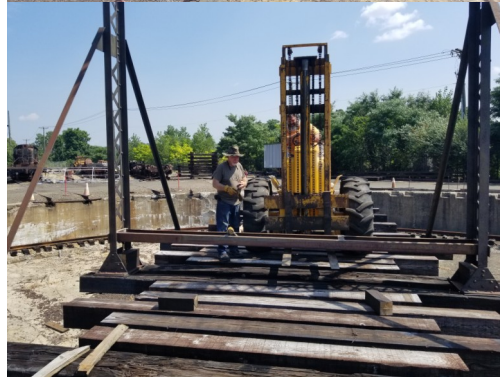
Left below: CMO Justin Chapin and Vice President Bill Wagner maneuver a metal beam between the bottom sides of the arch. Because of how the arch is constructed, it must be braced towards the bottom to prevent it from collapsing in on itself when the crane lifts it. Photo by Alden Burns.
